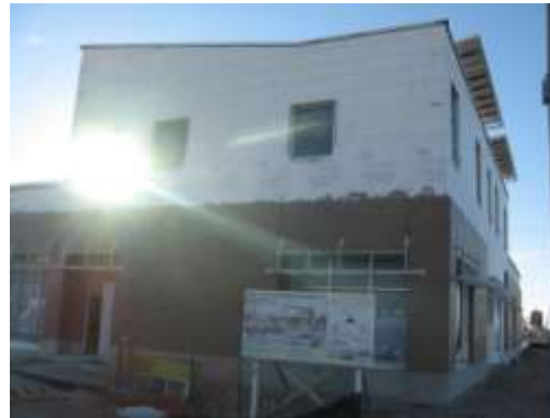
7 kW Photovoltaics (roof, top right) on Sunchips Business Incubator
